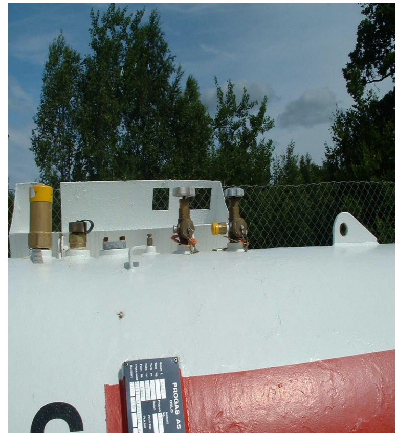
Standard tankarmatur for 2,4m 3 lagertank
